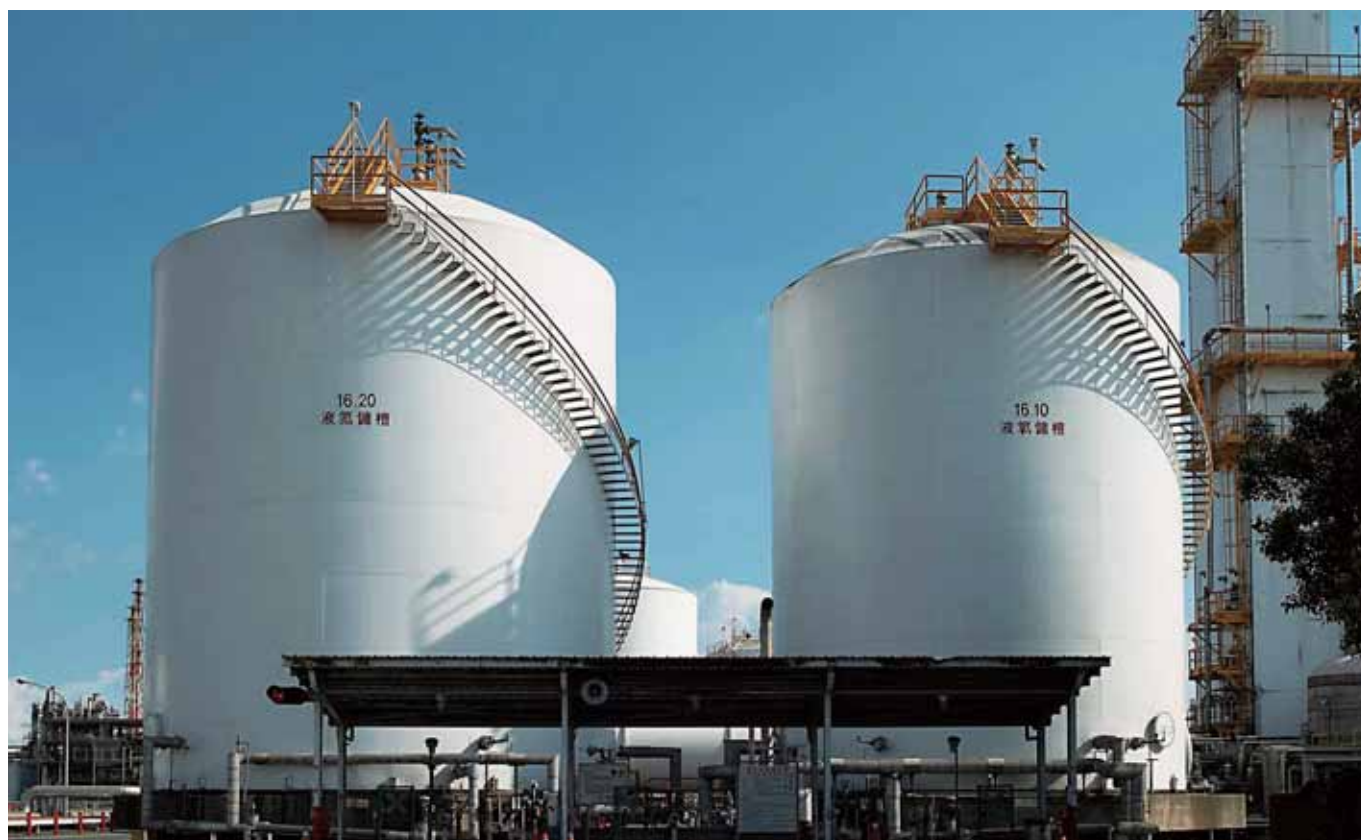
LN2 and LO2 storage tanks at the air separation factory of Yongan LNG Plant
