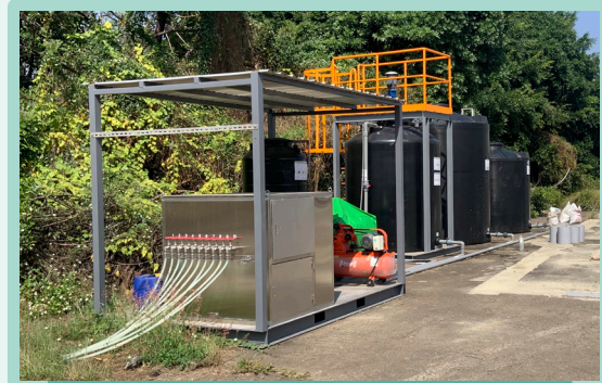
Automated chemical injection system
