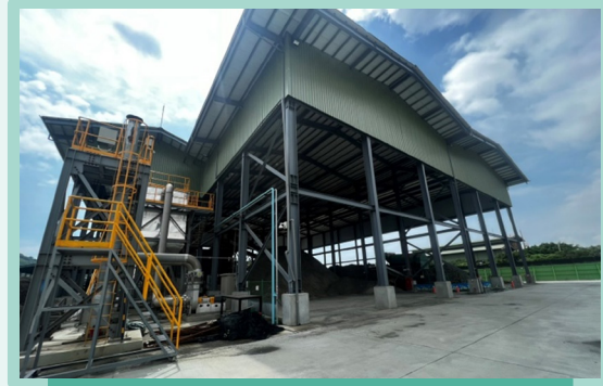
Thermal treatment equipment site
