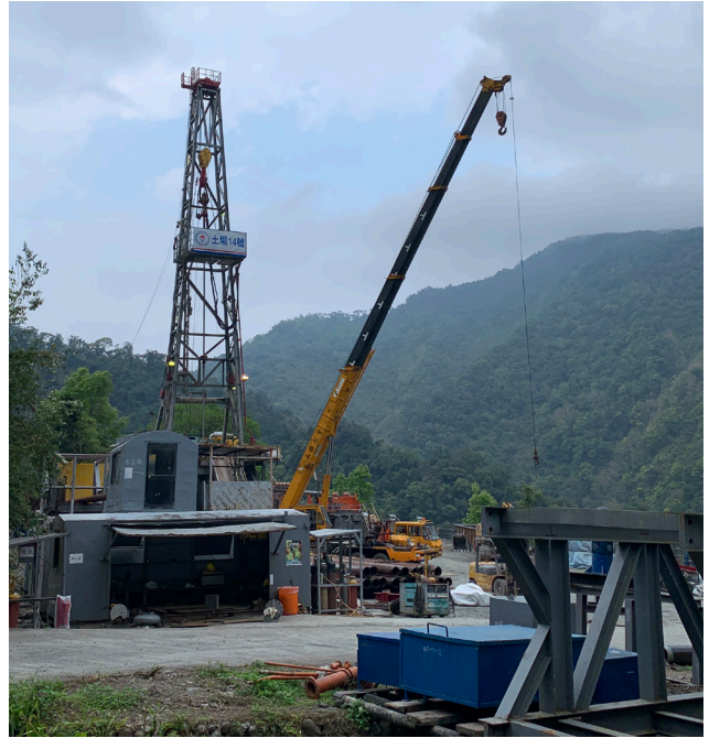
The geothermal drill site in Tuchang, Yilan, is located in a remote mountainous area
