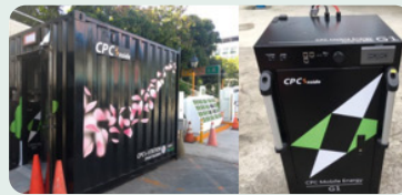
Taoyuan Jiadong Station: Test soft carbon energy storage system
