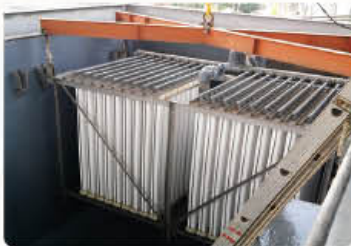
Membrane Bioreactor (MBR)
