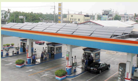
The PV system at Linluo Station
